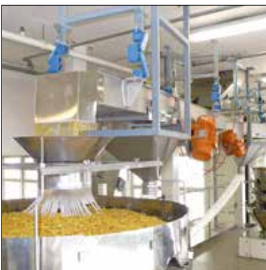
Pasta conveying chute suspended on HS mountings
