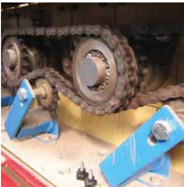
Tensioner devices for chain drives on loading stations
