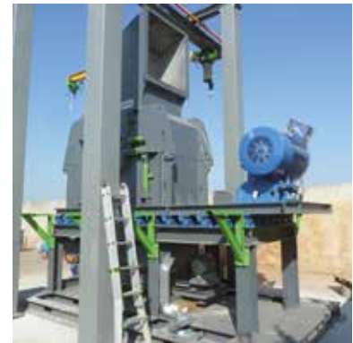
Motorbase in industrial shredder
